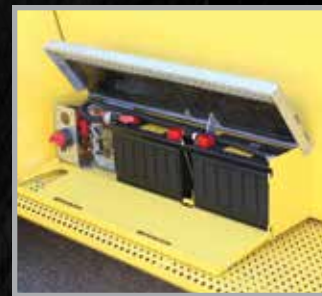
Battery box with Quick Disconnect Switch.
